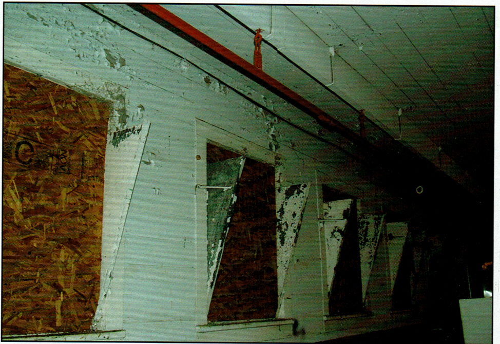
This photo shows a carrier system above the old stalls that probably was used to feed the cows. The patients at the mental hospital worked in this barn from 1923 till the operation was moved in the Fifties.
